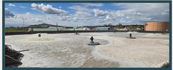
Splasher Aerators in Lagoon 1
